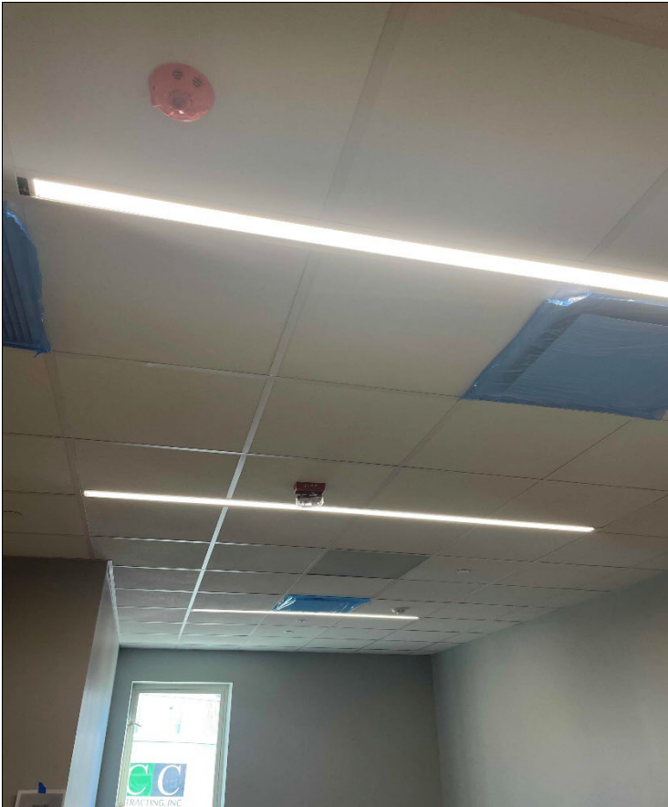
ACT Installation in Fire Prevention Room 115
