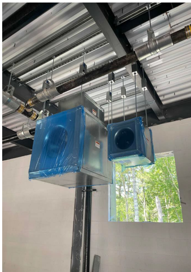
Exhaust fans installed on the apparatus bay mezzanine
