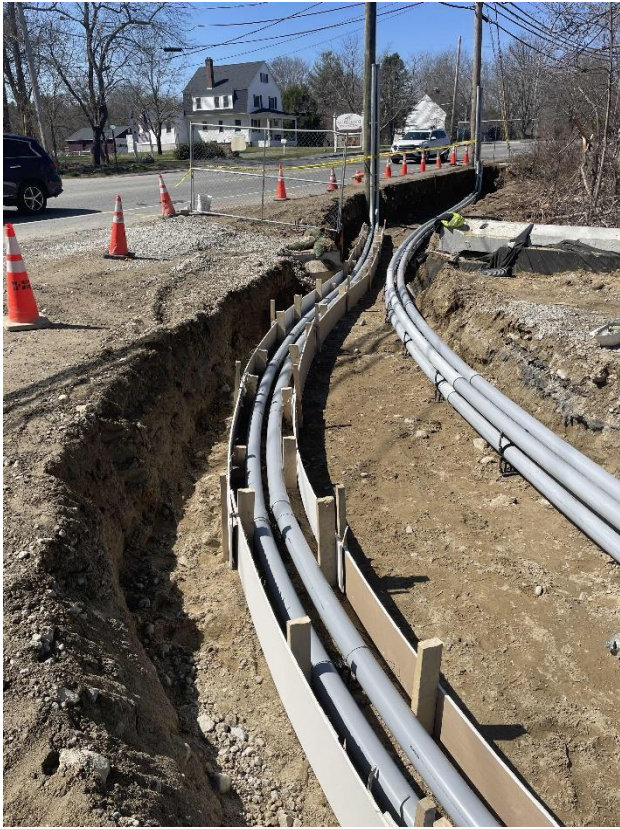
Primary Electrical & Communication Ductbank
